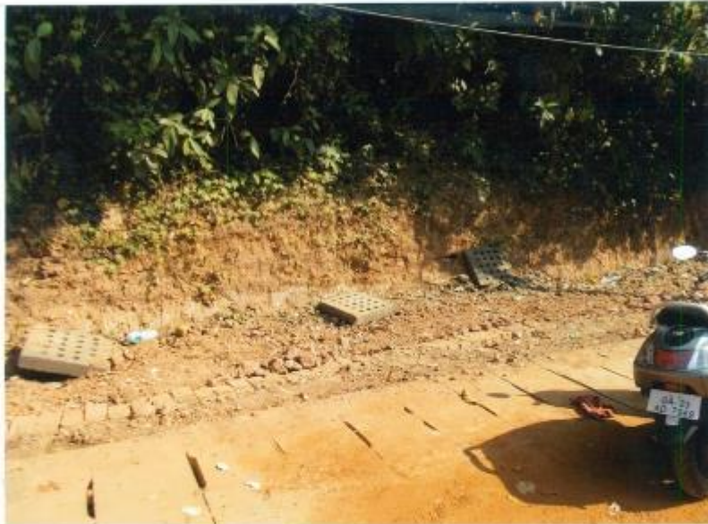
Road widening area on the side of Mary Immaculate Church road leading to Cortim down below
