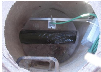
Sensor on Sewage Pipe
