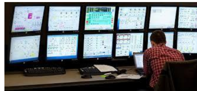
Water SCADA system
